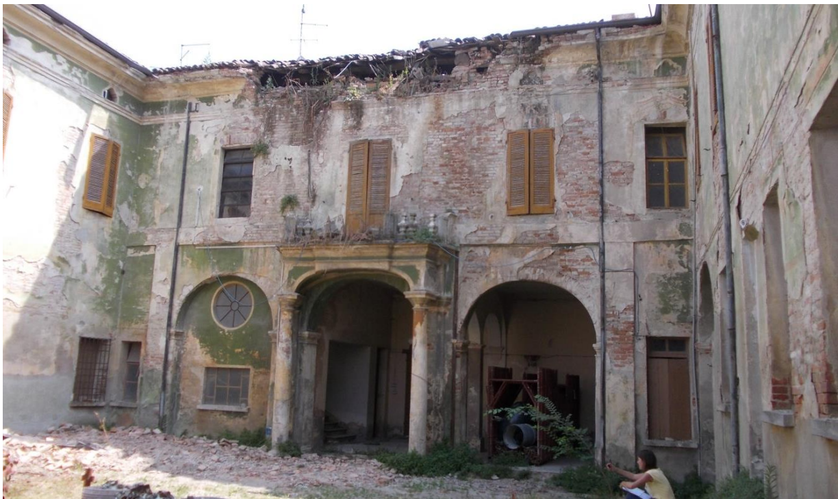
Figure 192-a. Seismic events 2012 in Emilia_ damage suffered by wall 4
