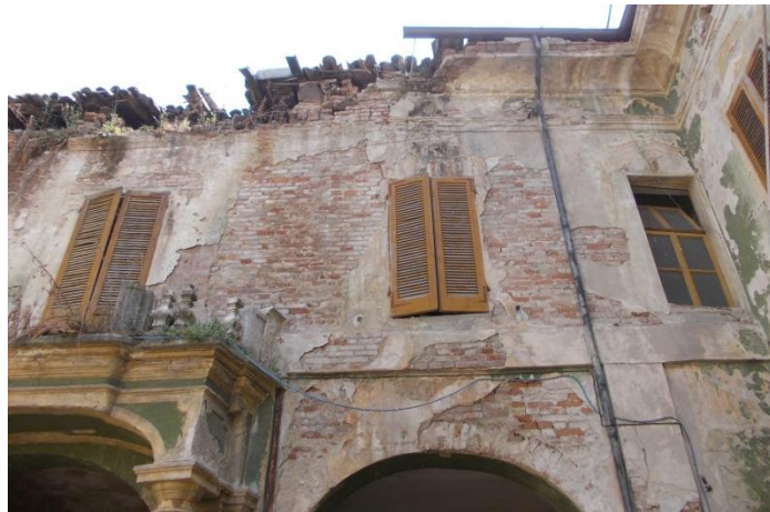
Figure 192-b-c. Seismic events 2012 in Emilia_ damage suffered by wall 4
