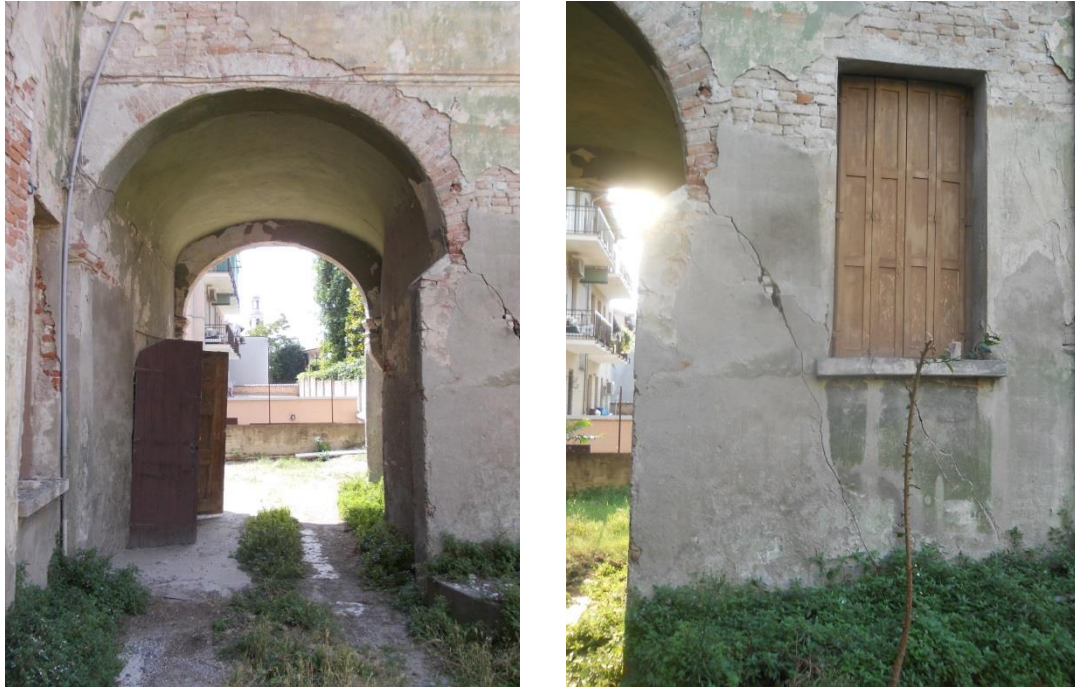
Figure 187-b/c. Seismic events 2012 in Emilia_ damage suffered by wall 3
