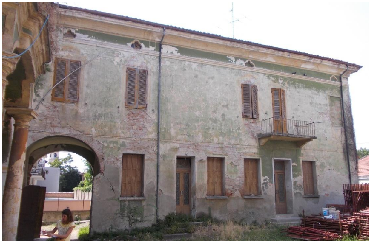
Figure 187-a. Seismic events 2012 in Emilia_ damage suffered by wall 3
